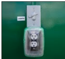
Weatherproof GFI receptacle and light switch
